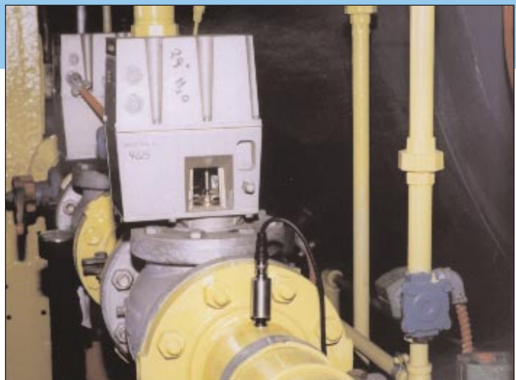
Valve flow / no flow condition monitoring.
